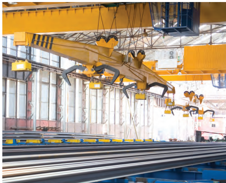
Material Transport Crane Applications
